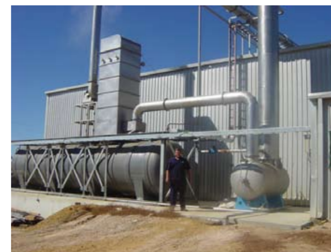
Odour treatment at Katanning
