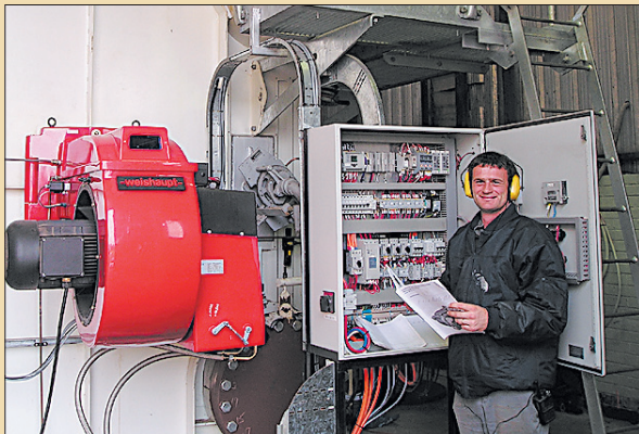
WAMMCO boiler attendant Adam Quick with the newly installed boiler equipment at Katanning
